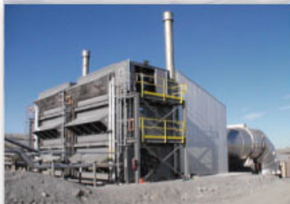
350,000 SCFM Indirect Fired Mine Air Heater - Artic Diesel
