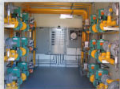
Custom Control Systems and Valve Train Design
