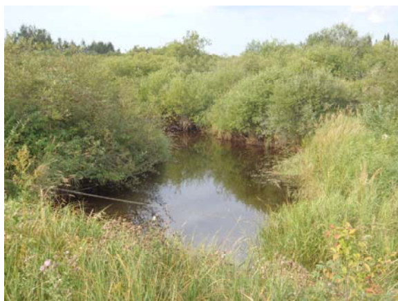
Picture 1: Culvert outlet on west side of the road, pool at basin of culvert.
