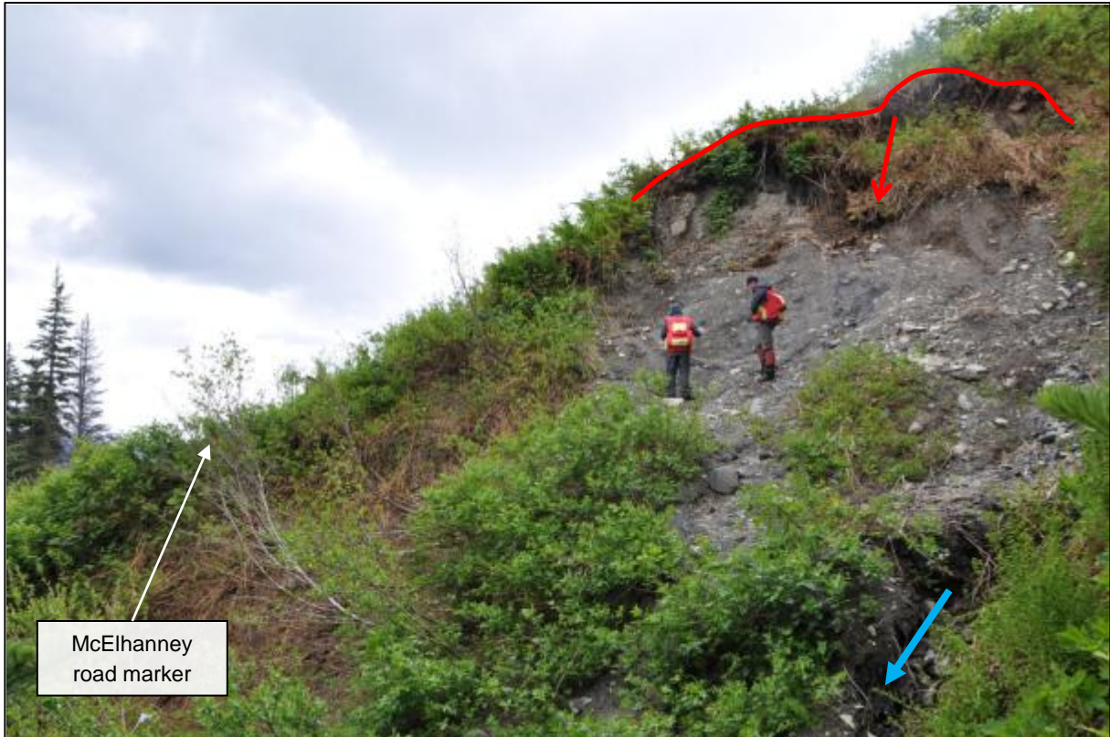
Photograph 22 North Treaty Upper Access Road – Looking upslope (south-southeast) from the left bank towards Km 1+480 at small landslide scarp (drawn in red) on the right bank of the creek. The small slump is 10 m to 15 m wide, 15 m to 20 m long on the slopes of a snowmelt channel. Soil is comprised of loose to compact sand (~50%) and gravels (~30%) with fines (~10-20%).
