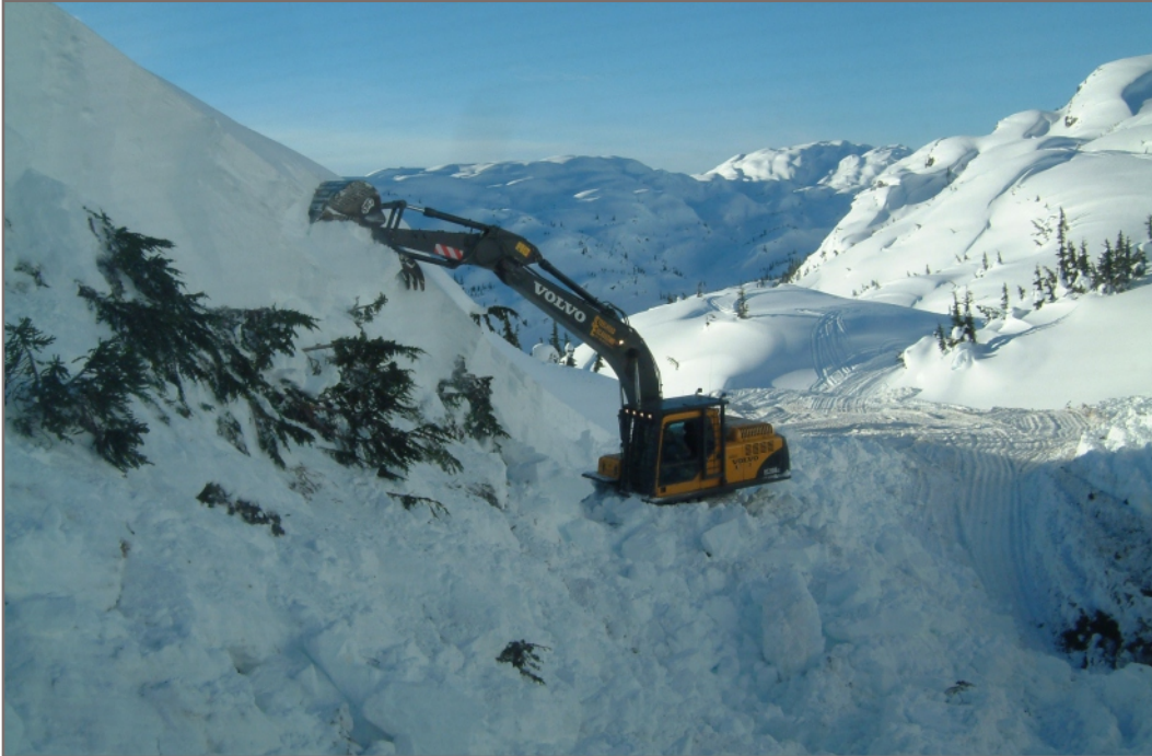
Photo 13: Photo from Brett Wildman of Nuna taken in the winter of 2009 showing a backhoe creating a drilling pad in the area immediately south of the Eskay Creek Mine.
