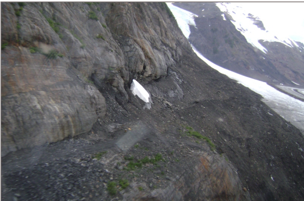
Photo 6: Looking to the northwest at a portion of the access road being constructed/ rehabilitated by Pretium to gain access onto the Knipple Glacier. The Knipple Glacier is visible in the distance on the right side of the picture.
