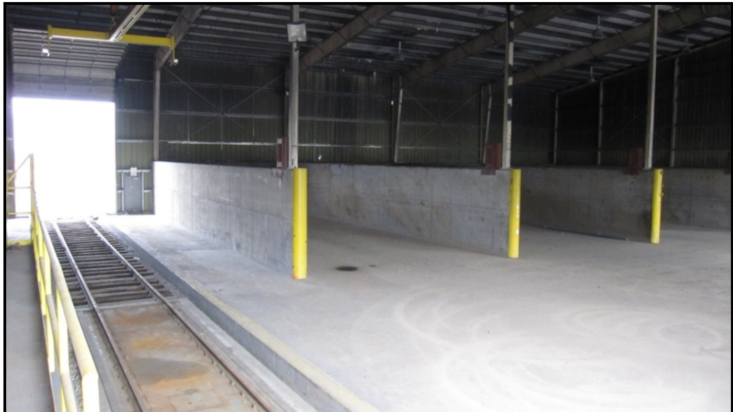
Figure 2.7 Kitwanga Facility Interior – Storage Bays and Rail Access
