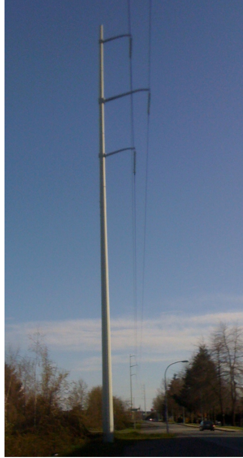
230 KV Monopole Line, Urban Setting Richmond, B.C.
