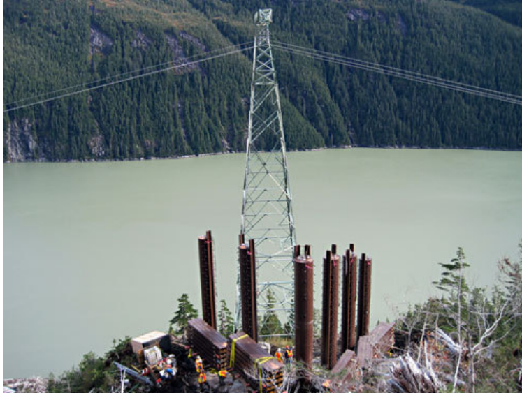
Figure 8.2 - 4 Diverter Structure In Alaska
