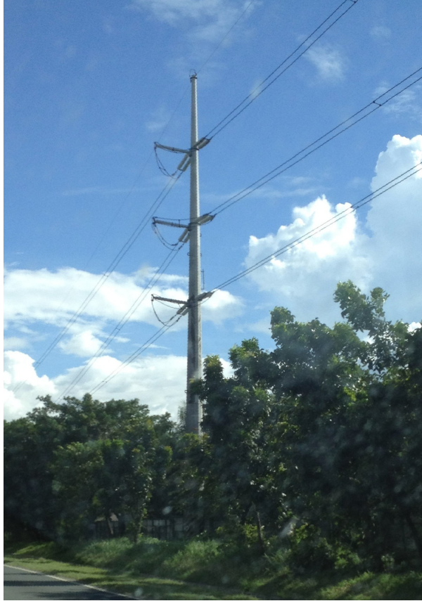
230 kV Monopole In-Line Dead-End
