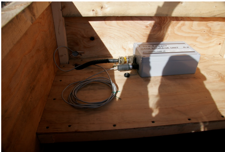
Photo 4: Datalogger connected to Thermistor within housing.
