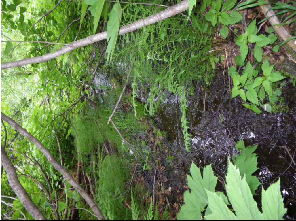
Stream/ILP: 2032 Site: 1 Image: 134 Comment: Downstream, Seepage at road crossing. 7/13/2009.
