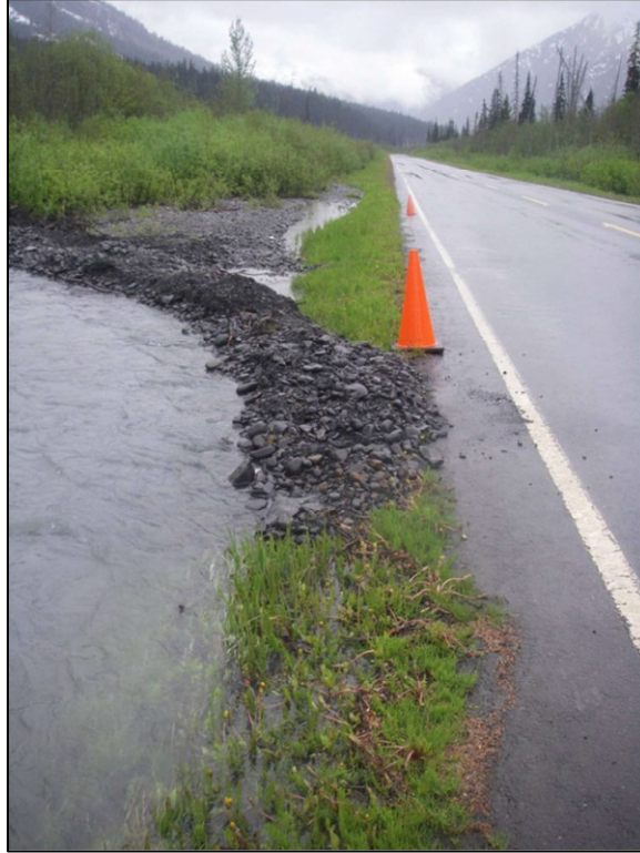
Plate 5.2-2. Water flow at road downstream of north culvert.
