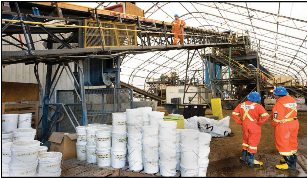
Onsite Processing Plant interior
