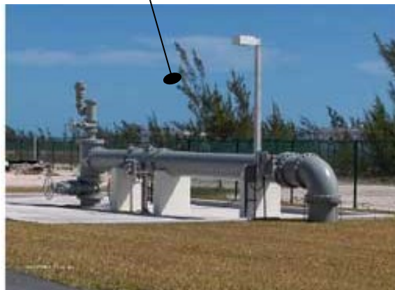
Injection well located at plant site
