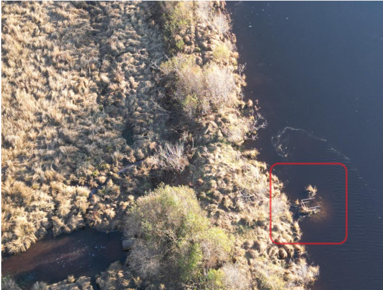
Figure 1. Drone image of degrading and plugged control structure, November 2023.
