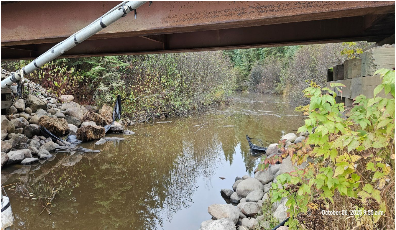
Photo 17. DC-02 Bridge – Facing upstream – large boulder and cobble substrate along edges of abutments. September 16, 2025
