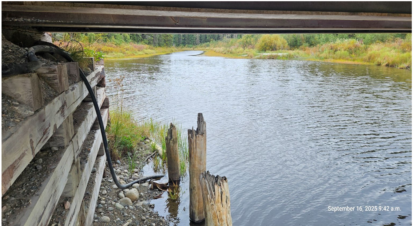
Photo 9. Reach 1 – Facing downstream – exposed gravel and coble along bridge abutment.
