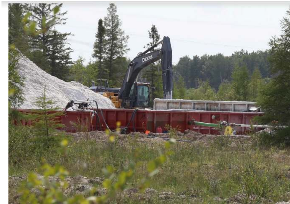
Figure 5. CWS sand extraction activities in a quarry site near Vivian MB Aug. 18, 2021
