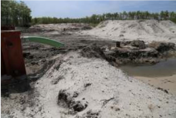
Figure 3a. Tanks near Vivian used to hold the water and sand drawn directly from the aquifer by CanWhite exploratory drilling, May 31, 2020
