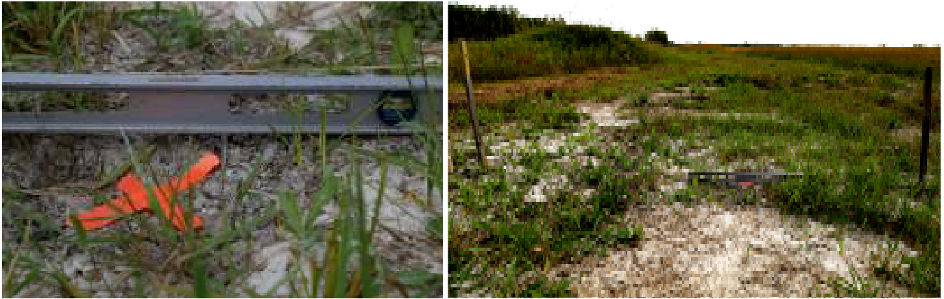
Figure 20 a and b Surface expression of abandoned sealed CanWhite borehole near Ross Manitoba in a slight depression (no mounding) with clay sealing on top of the cut off borehole.
