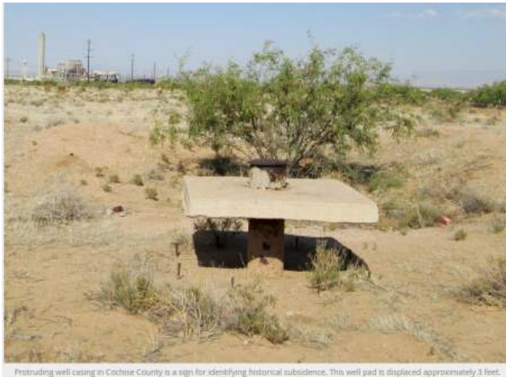
Protruding well casing in Cochise County is a sign for identifying historical subsidence. This well pad is displaced approximately 3 feet.
