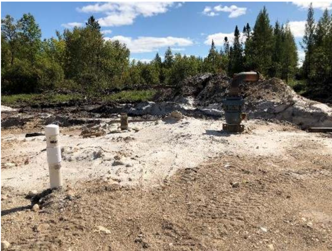
Figure 17. CanWhite boreholes with no grout or sealing around the casing near Vivian spring, 2020.
