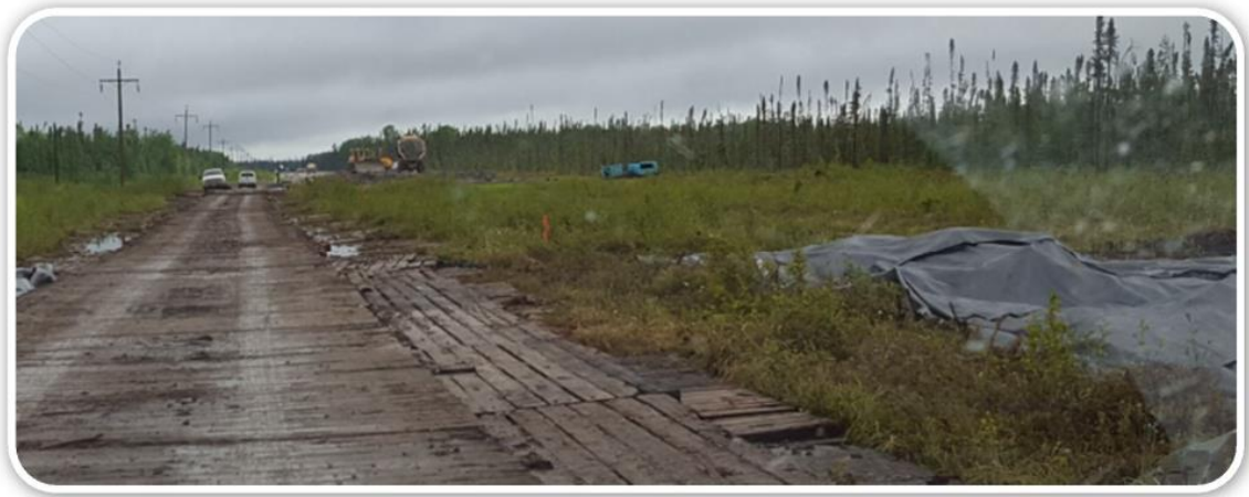
Use of Use of Swamp Mats to access construction sites in frost free conditions
