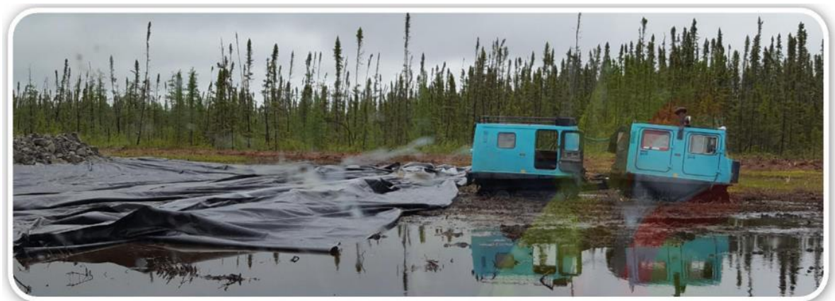
Russian Hagglund working ahead of subgrade placement used to place sewn geotextile
