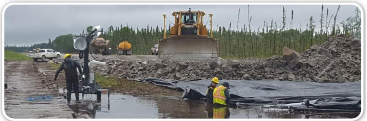
Typical condition of placement of muck in frost free conditions through boggy Terrain
