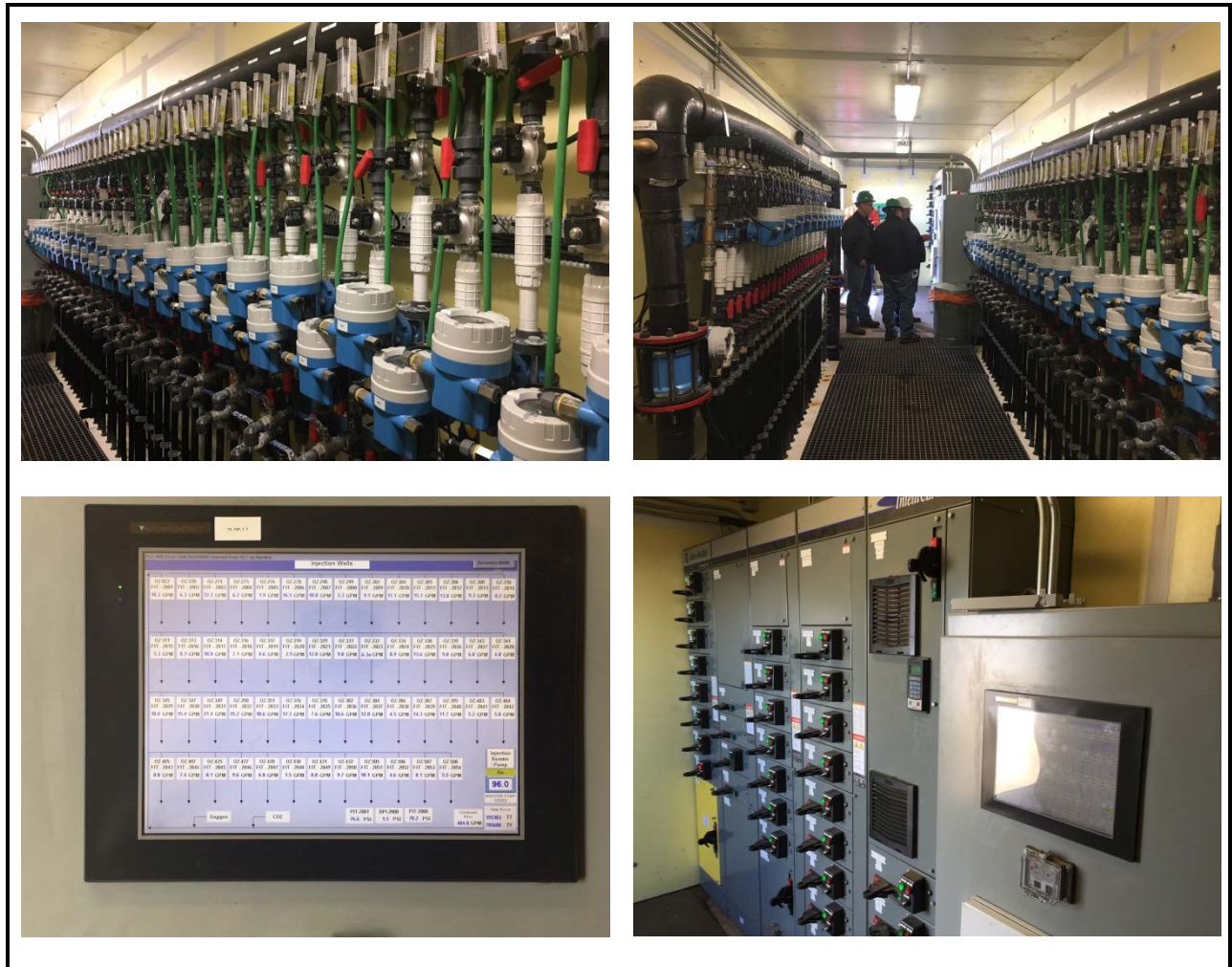
Figure 2.10: Inside a Typical In Situ Recovery Pumphouse
