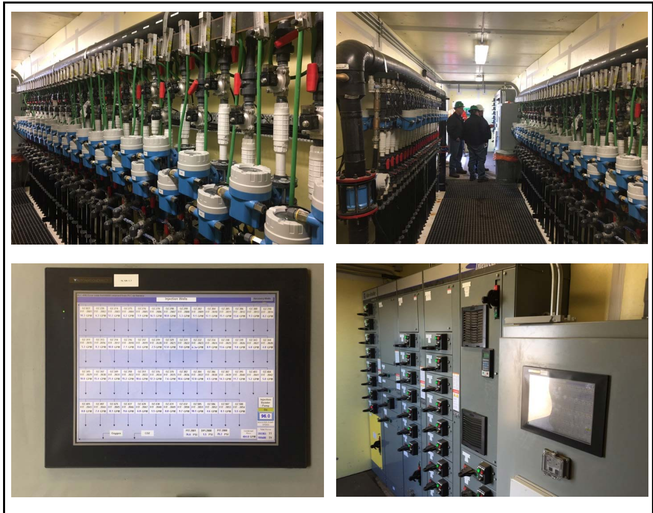
Figure 2.11: Inside a Typical In Situ Recovery Pumphouse
