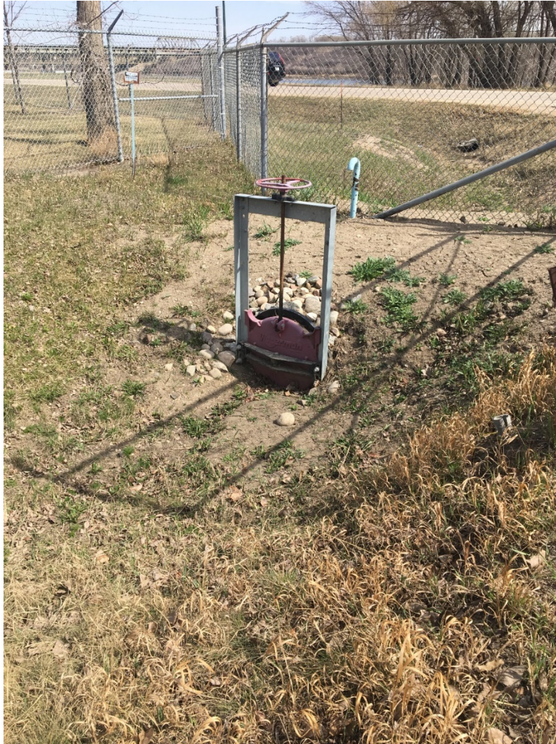
Photo 1 Example of manual operated shut-off as a control gate from SaskPower's Queen Elizabeth Power Station located in Saskatoon, SK.
