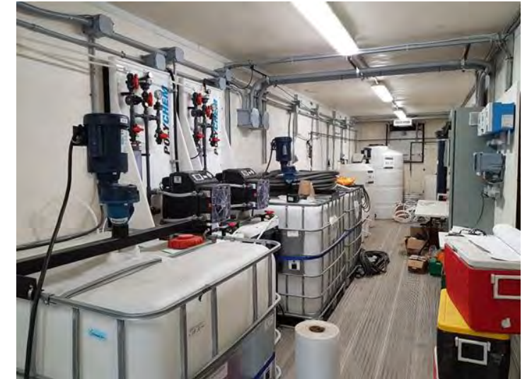
Water treatment facility
