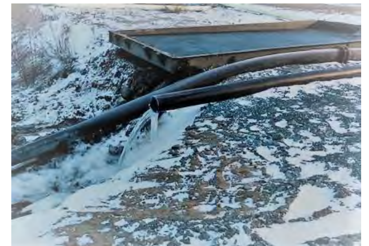
Clear water leaving the treatment facility
