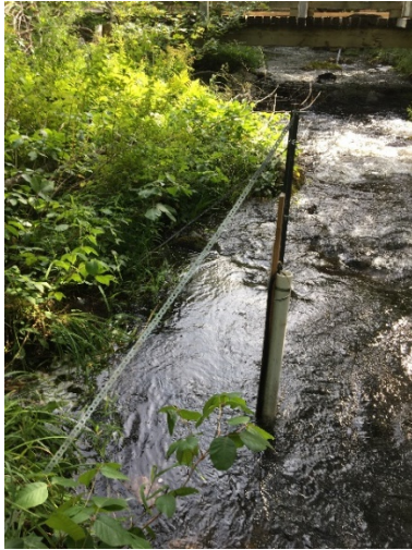
Photo 1: Hydrometric Station Installed at SW2
