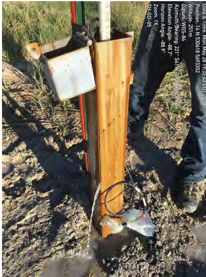
Figure 2: TH-GD-05 with a crack in the metal casing visible in the middle of the picture. Water leaked through after the PVC standpipe was opened, but stopped leaking after the PVC standpipe was re-sealed.
