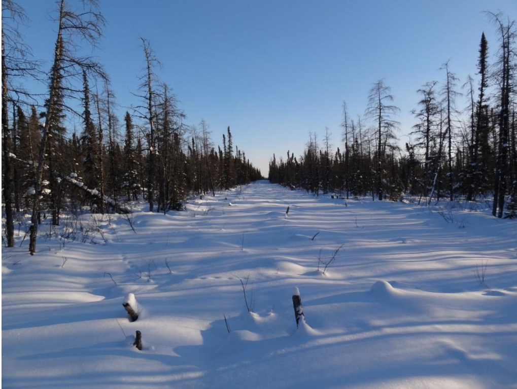
Photo 8: Exploratory clearing completed along proposed All-Season Road alignment approaching Manto Sipi Cree Nation
