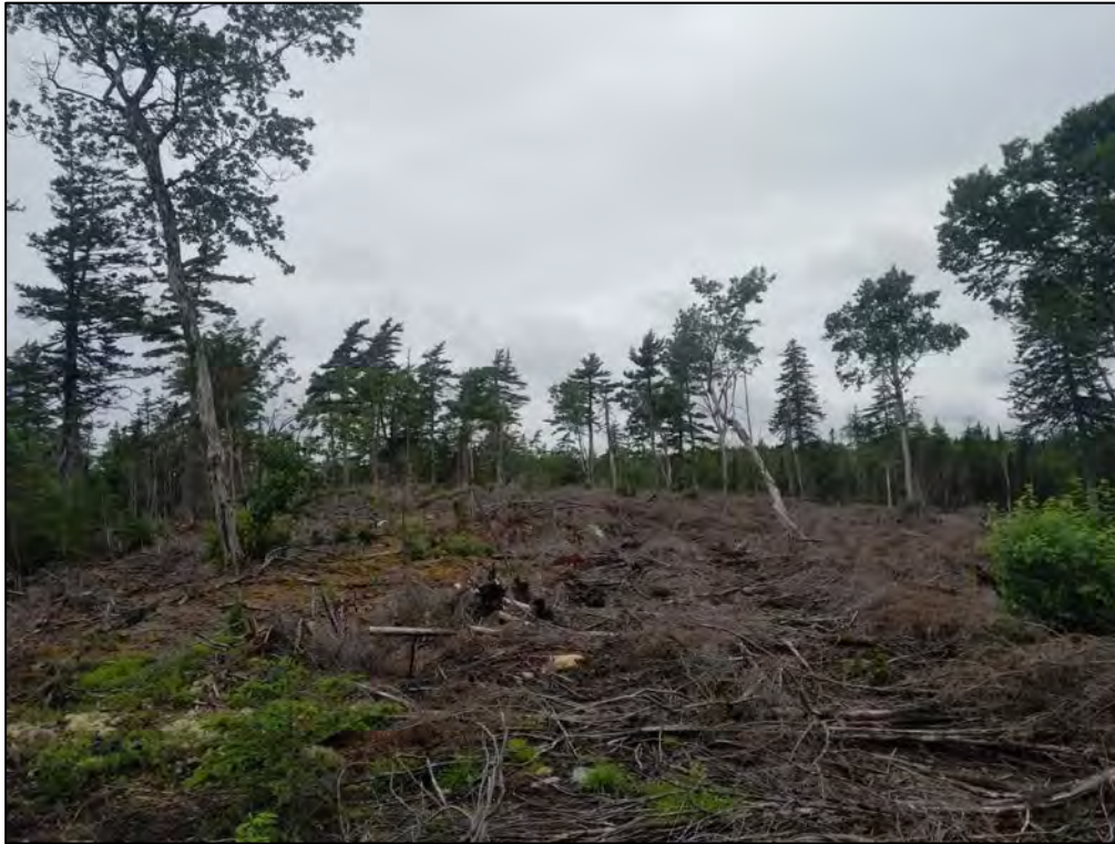
PLATE 15: Recent tree clearing operations, avoiding the surrounding low wet areas with standing water. Facing southwest; July 23, 2019.
