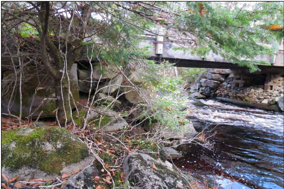
Plate 6: West River Sheet Harbour crossing, exhibiting some disturbance; facing north. November 13, 2015.
