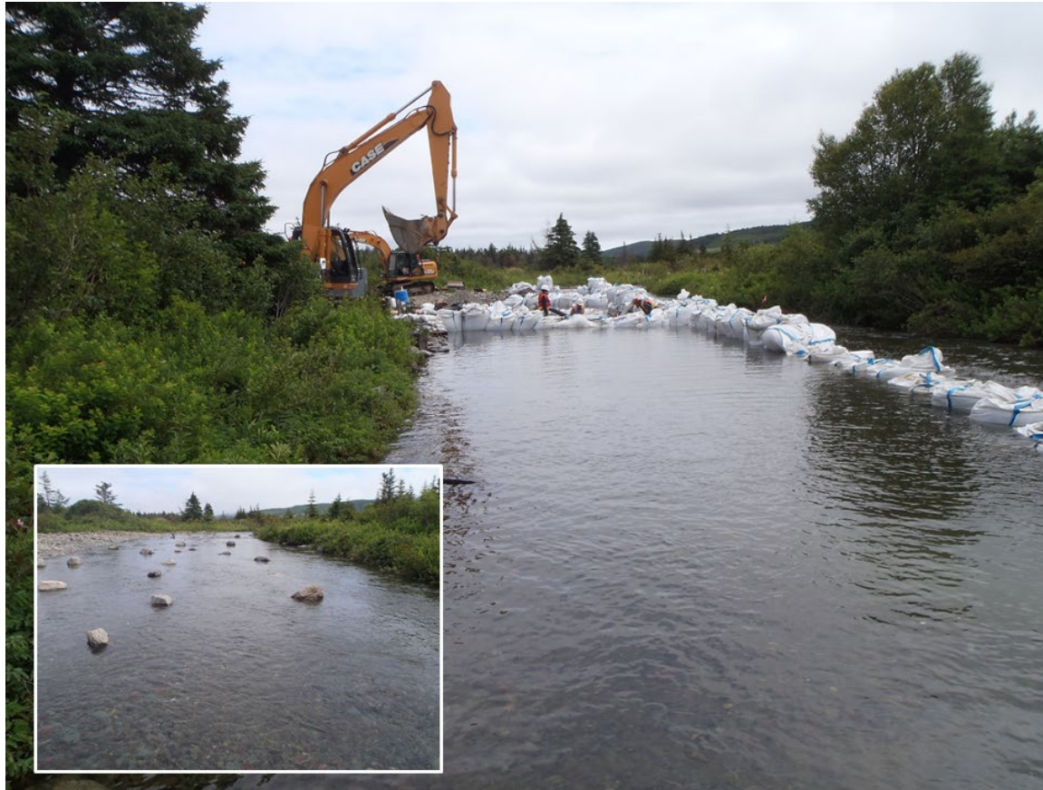
Figure 37: Typical in-river Atlantic Salmon spawning/rearing habitat isolation and construction. Completed habitat inset.
