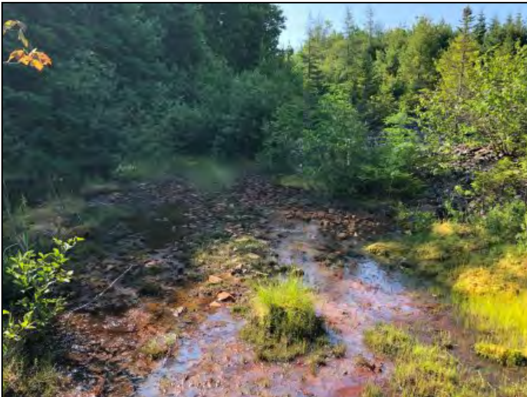
Seepage from the base of the dam stained red looking east
