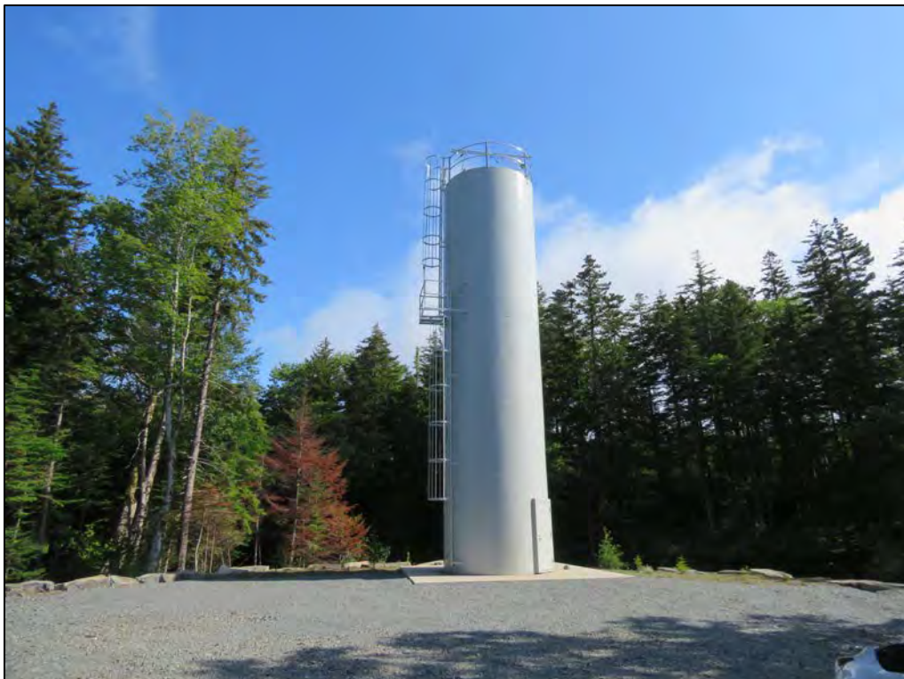
PLATE 4: Automated lime dosing station on the west bank of the Killag River. Facing northeast; July 22, 2019
