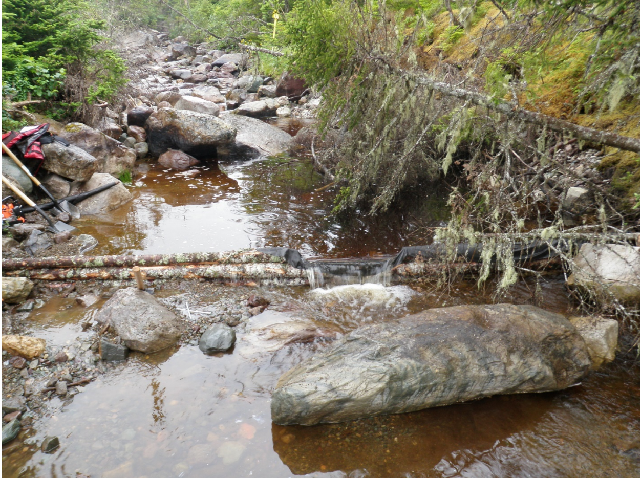
Figure 31: Small low-head barriers being installed in a stream to add pool habitat and complexity after hurricane damage
