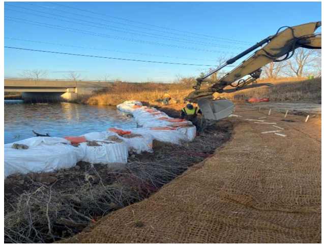
Photo 14: During construction Indian Creek (2022). Approximately 1 km northwest of Lower Baseline at Tremaine Road. Downstream left bank rehabilitation. Facing upstream (southwest)
