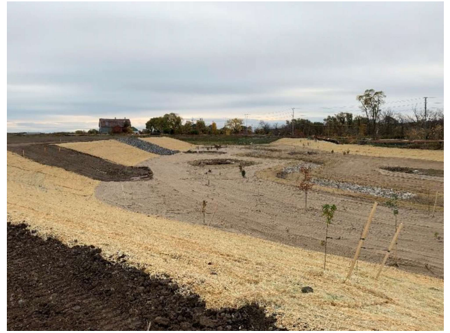
Photo 8: During construction Tributary A. South end of realignment facing Tremaine Road (southeast). Off-line floodplain
