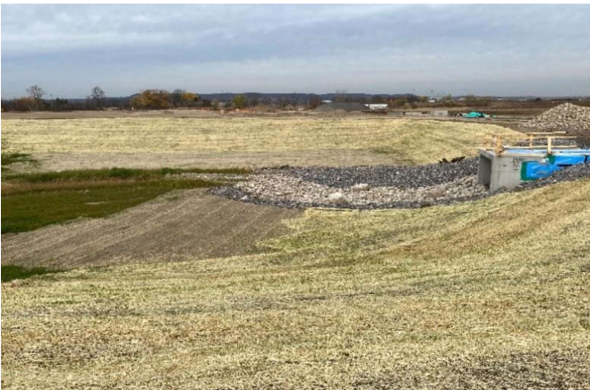
Photo 5: During construction Tributary A (2022). At new culvert downstream of existing main line. Facing west.
