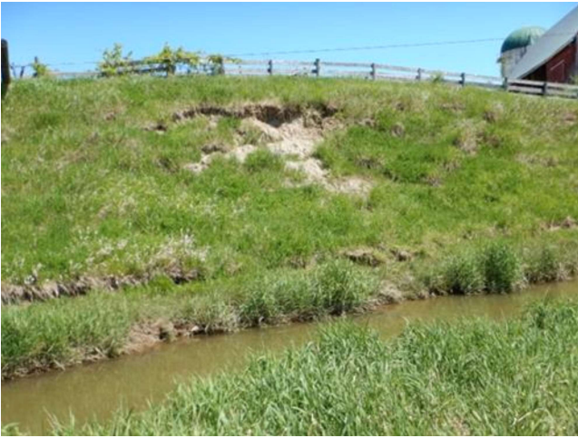
Photo 13: Pre-construction Indian Creek (2014). Approximately 250m downstream (east) of Tremaine Road. Facing the downstream left eroded bank.
