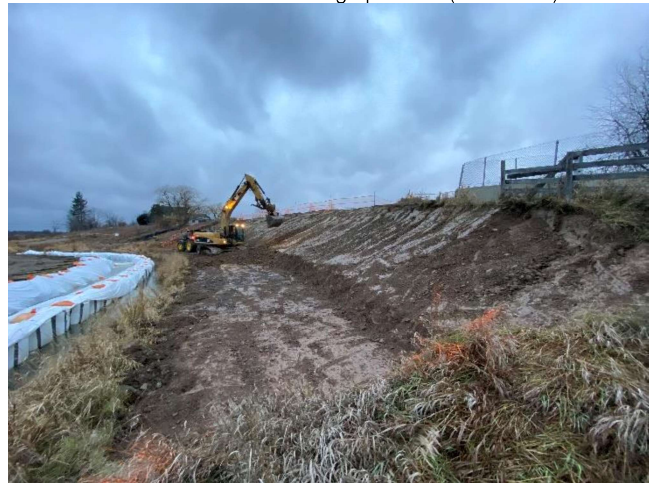
Photo 16: During construction Indian Creek (2022). Approximately 200 downstream (northeast) of Tremaine Road. Regrading downstream left eroding bank. Facing upstream (southwest).
