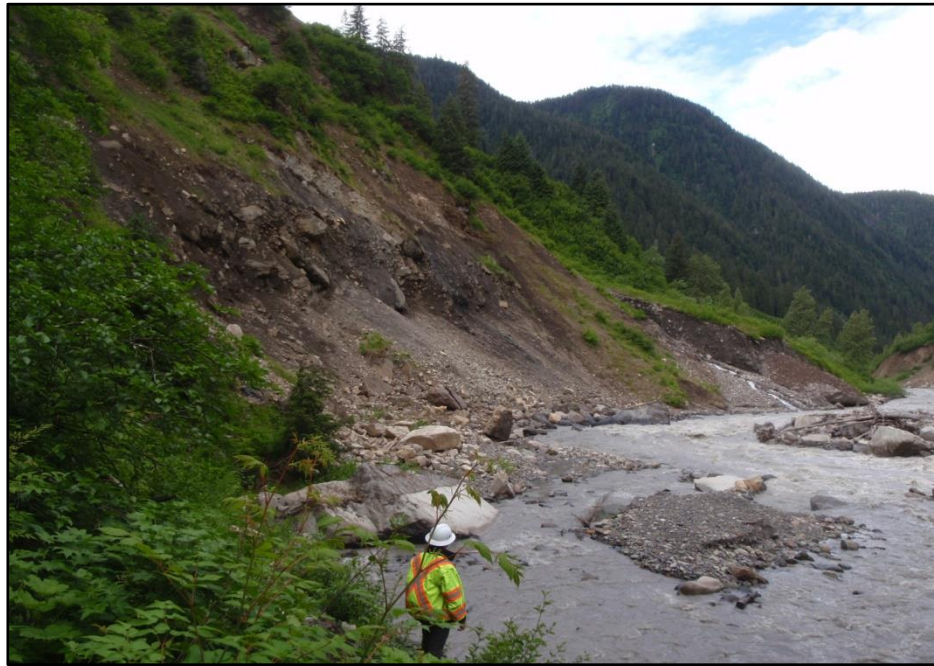
Figure 4-4 Looking along the downstream section of the channel bend's left bank between Stations 4+600 and 4+820
