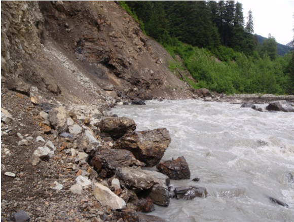
Photo 5: Looking upstream along bedrock controlled channel bend with eroding & over-steepened hillslopes in the vicinity of Stn 4+700. June 13, 2017
