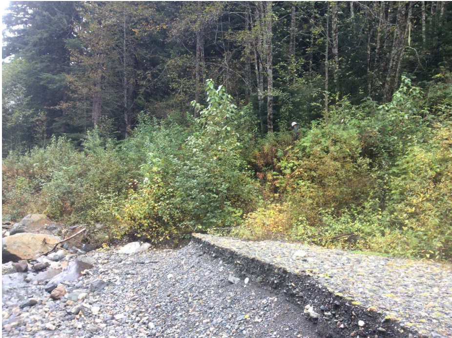
Figure 31. View of a washed away section of road near road station 2+880.
