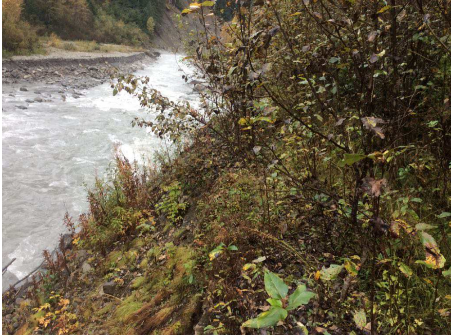
Figure 41. View from the north bank of Bitter Creek, near road station 3+450, looking downstream.
