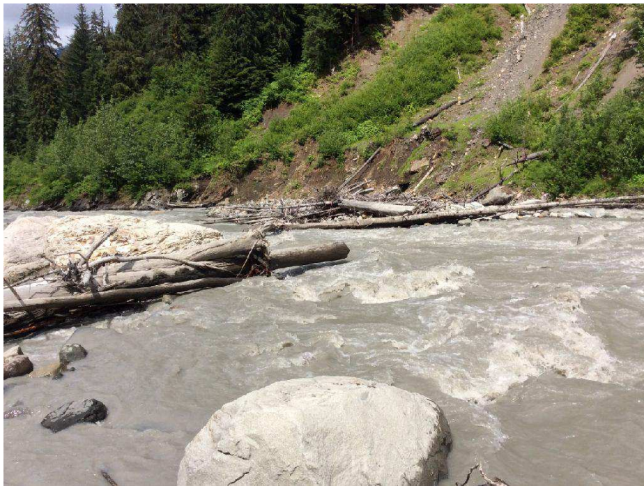
Figure 112. View of a small log jam from the south side of Bitter Creek, near road station 4+115.
