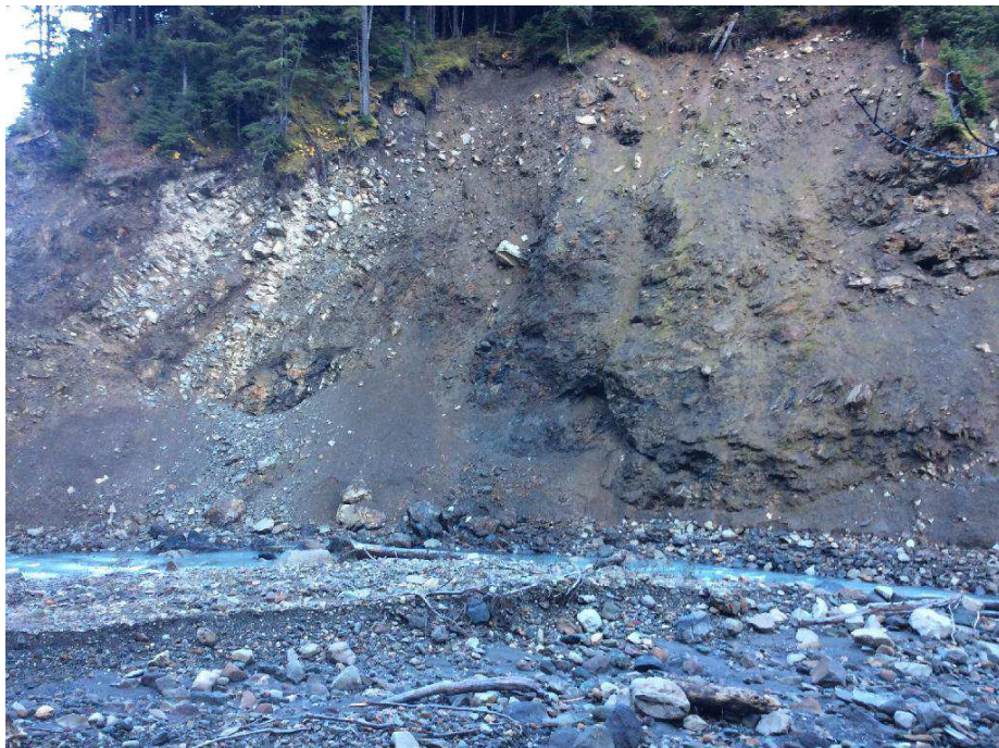
Figure 152. View from a gravel bar on the south side of Bitter Creek, near road station 4+660, looking towards the north bank.
