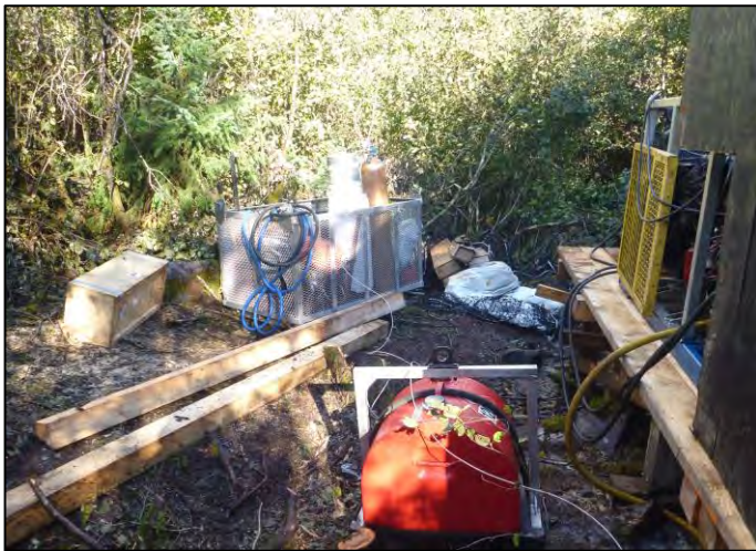
PHOTO 59 MW16-002 Nitrogen gas setup
