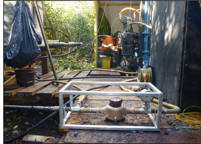
PHOTO 58 MW16-002 Flowmeter Assembly
