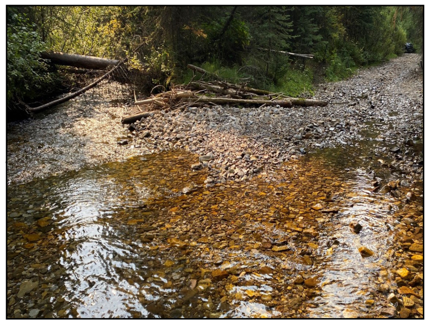
Photo 2 Right bank of truck ford and road prone to flooding during high water events.
