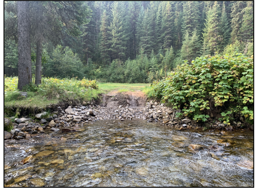
Photo 2 Erosion on right bank of truck ford.
