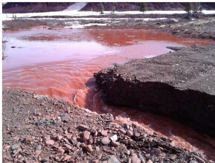
Figure 2. Closeup of breach at the SP3 SE corner, with water flowing into SP3.
