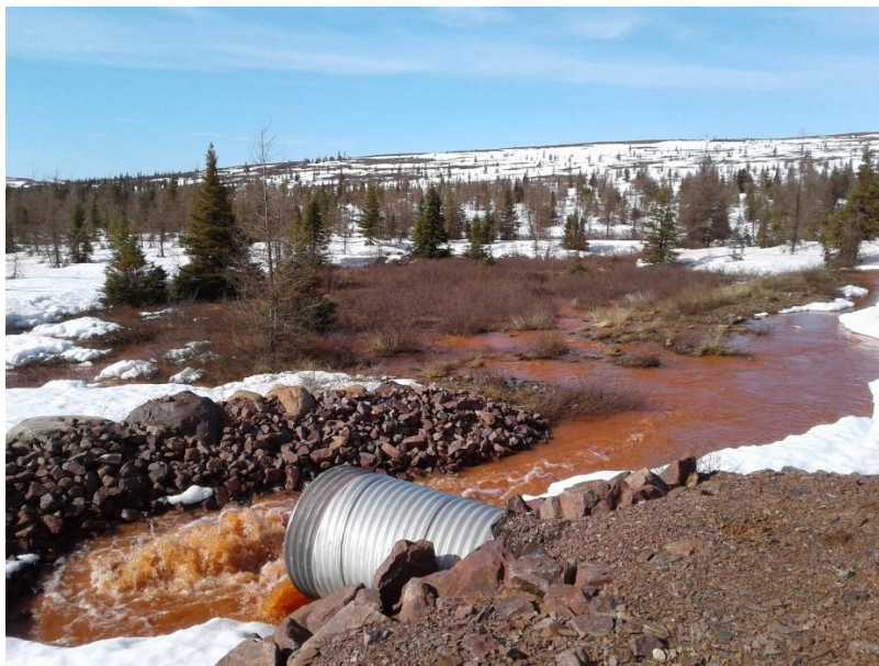
Figure 4. Water flowing from culvert into adjacent wetland.
