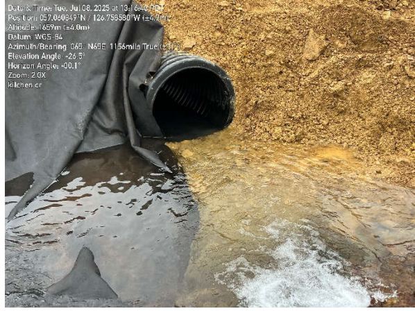
Plate 008: Photo KW009. Full barrier, 10m falls, full barrier to Plate 008. Geofabric installation at inflow of 900mm culvert at site KN001.
