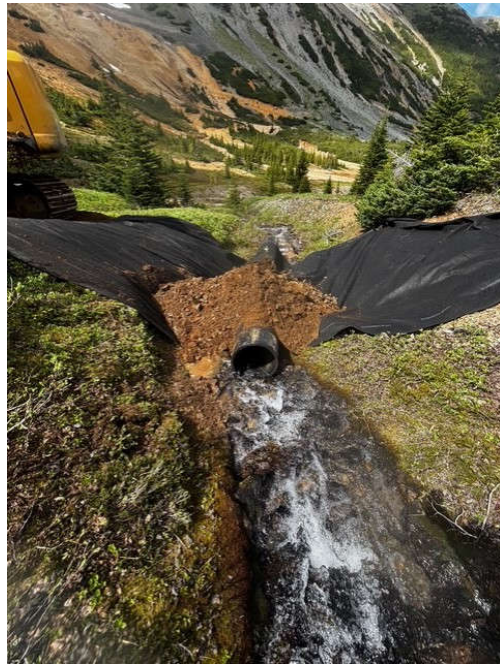
Plate 018: Installation of geofabric and 600mm round plastic culvert at temporary crossing KN003.
