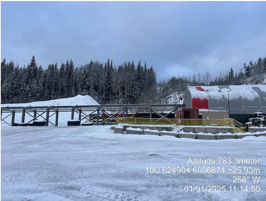
Appendix Photo A-2. Monorail system and hoist house construction progress on January 1, 2025.
