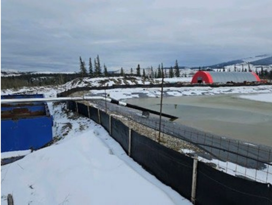
Appendix Photo A-1. Dewatering piping from the underground to the primary pond at the decline site on March 29, 2025.
