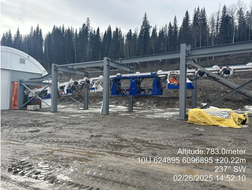
Appendix Photo A-3. Hoist house and monorail system construction progress to February 26, 2025.
