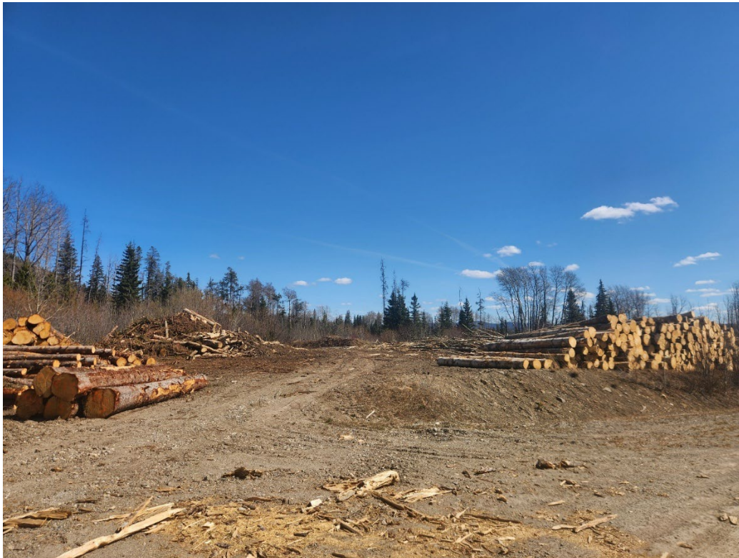
Appendix Photo A-10. Timber from tree clearing activities at the shaft site April 24, 2025.
