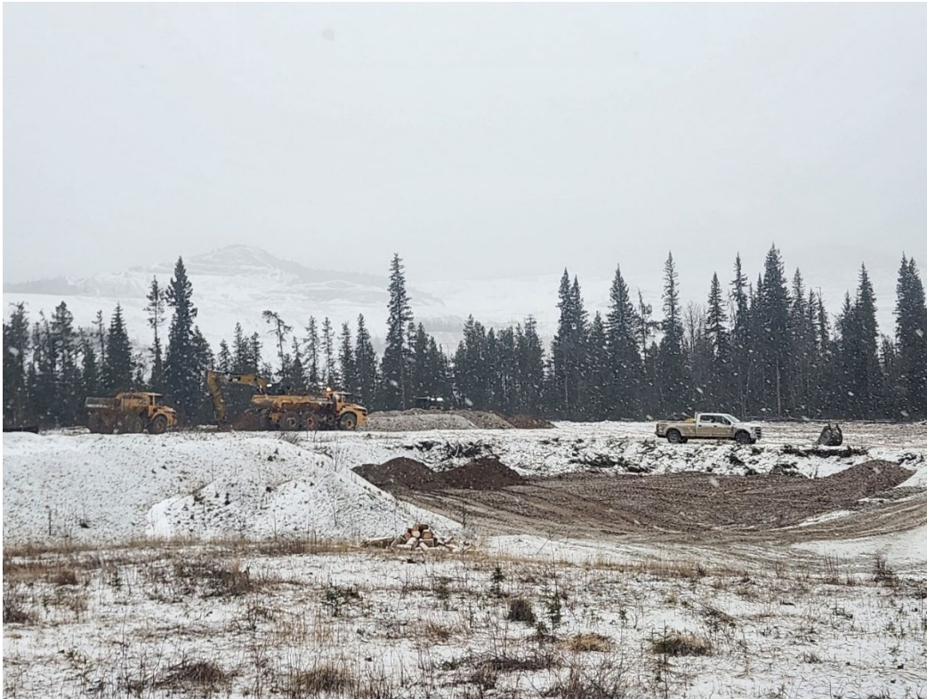
Appendix Photo A-5. Tree clearing activities at the decline site on March 12, 2025.
