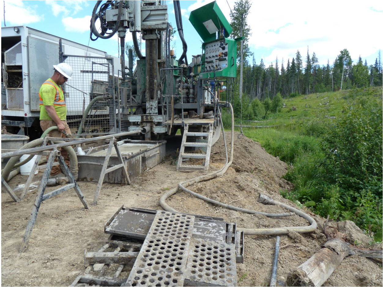
Figure 3 BH - 04. Note approx. 5 ft of road fill on top of natural ground
