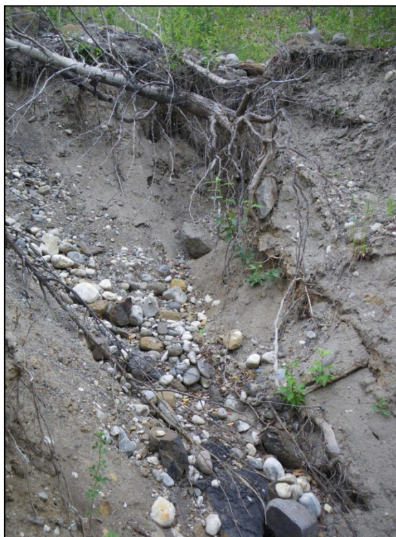
Plate 4.3-4. Soil erosion was occasionally recorded on constructed slopes.
