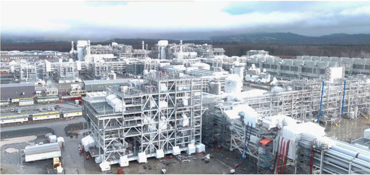
PHOTO 4: LNG FACILITY – VIEW OF THE LNG TRAINS 1 AND 2 TO THE NORTH (MARCH 2025)
