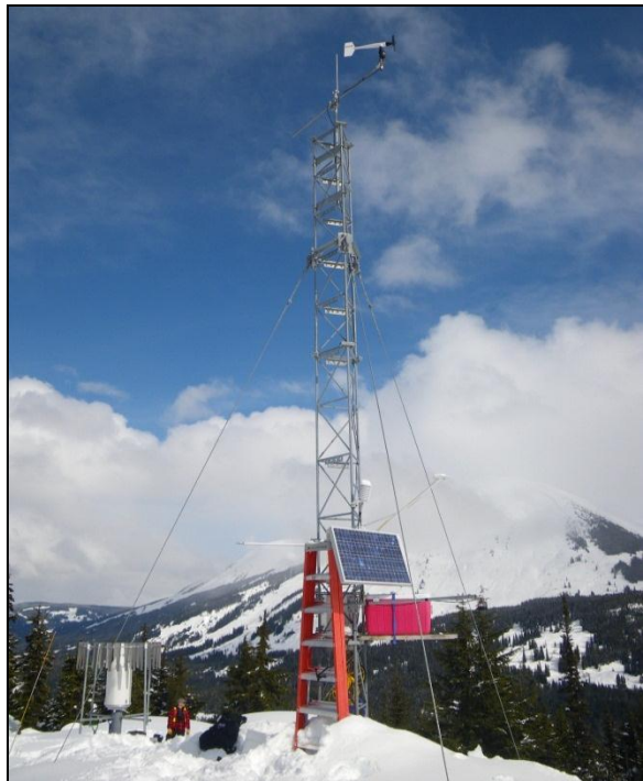
Plate 7.3-2. Scott Creek meteorological station, March 2012.
