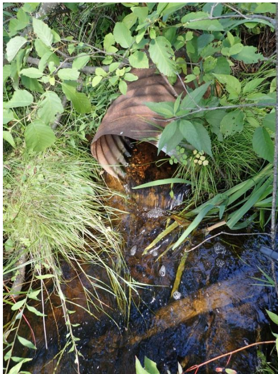
Figure 3.1.2-6. Corrugated steel pipe conveying Blackwater Creek Tributary 2 beneath a forestry road in Reach 2, approximately 1.25 km upstream from Normans Road.
