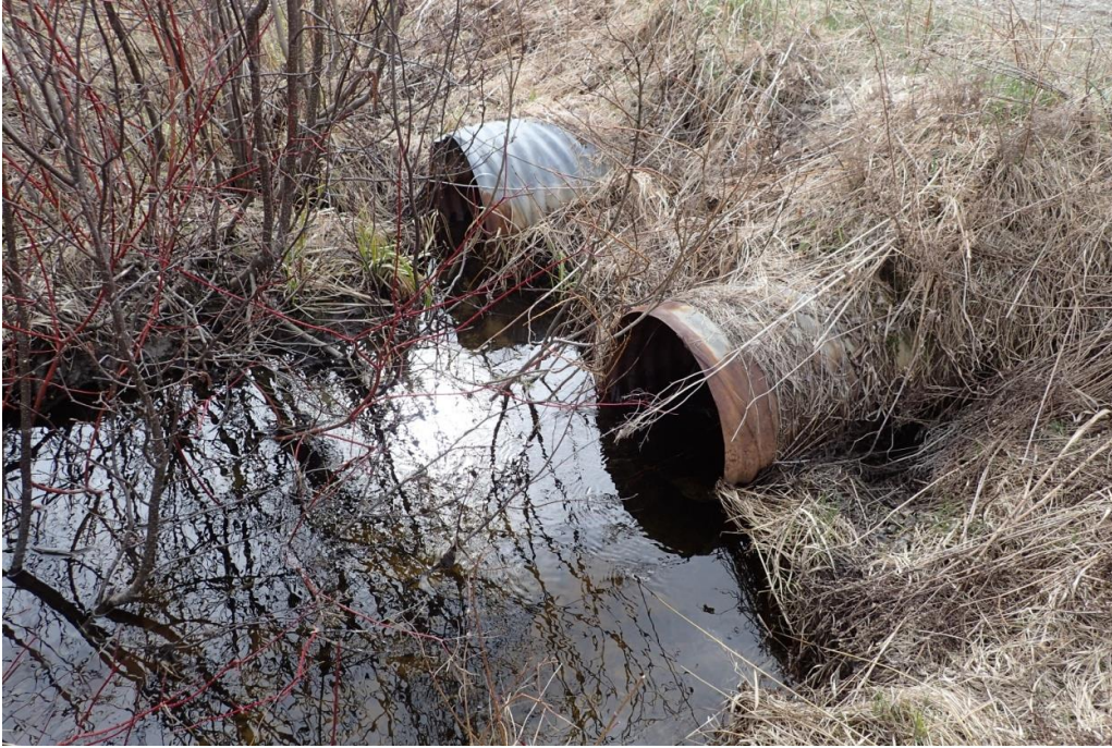
Figure 3.1.2-5. Corrugated steel pipes that convey Blackwater Creek Tributary 2 beneath Norman's Road. Most of the flow is conveyed by the culvert on the right.
