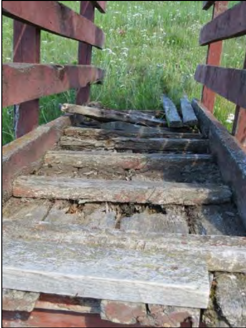
Photo 7. Cattle-handling infrastructure needing repair
