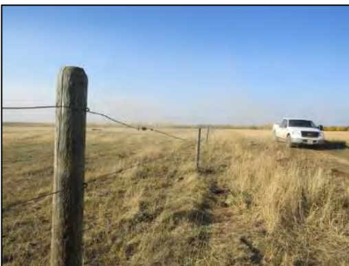
Photo 5. Existing fencing needing repair
