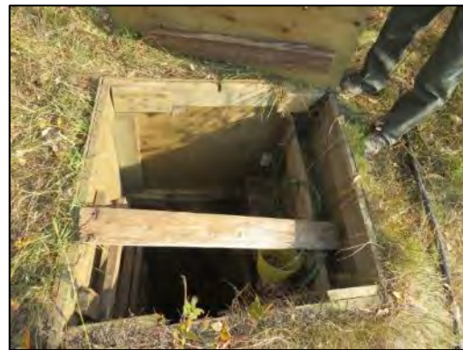
Photo 10. Dry well at dugout #1
