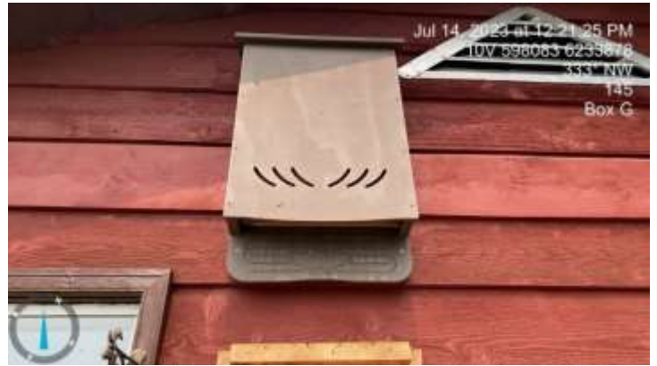
Photo 6: A large amount of guano was found at BAT_145_G on 14 July. Wooden ledge beneath box intended to capture guano in lieu of a screen.
