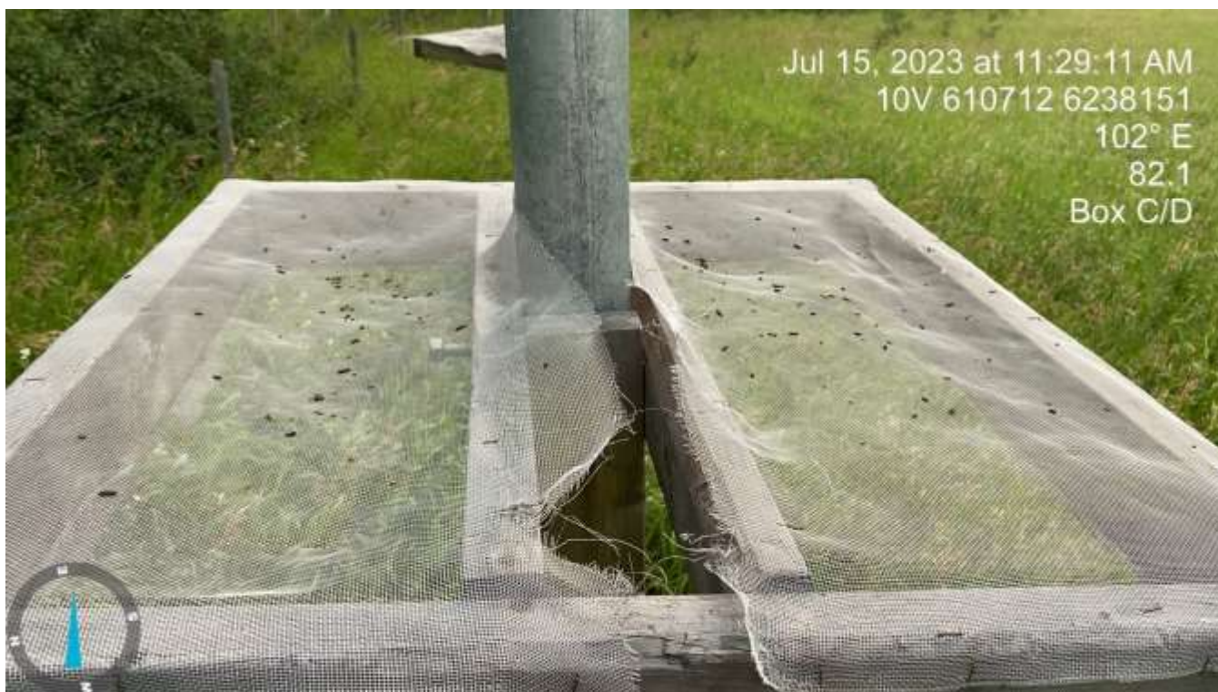
Photo 12: Example of a 'Moderate' quantity of guano beneath BAT_82.1 C/D on 15 July 2023.
