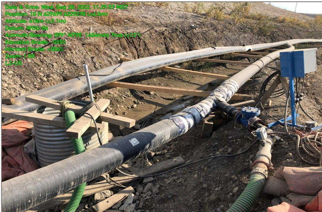
Photo 22: L2-US sample location, September 2022.
