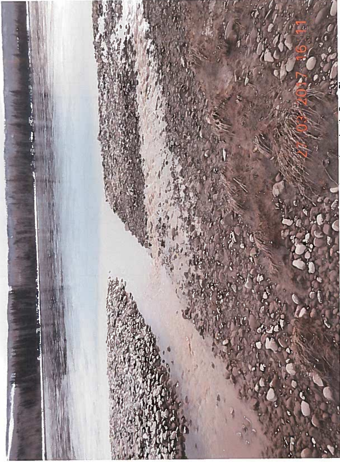
Figure 4: Sediment laden water exiting Unnamed Creek 3 culvert and entering the Peace River
