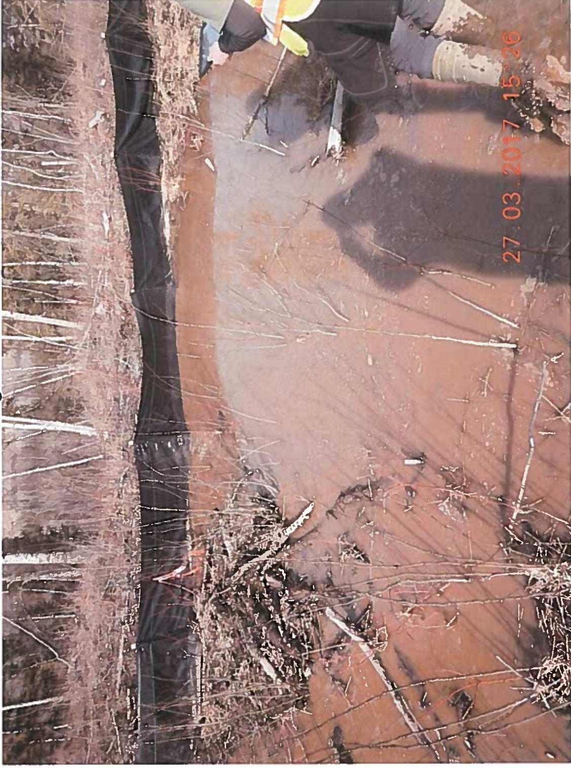
Figure 7: Sediment Laden water leaving Area A work area
