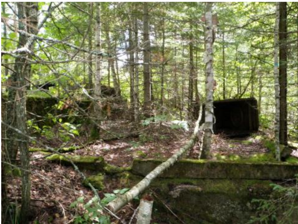
Figure 15: View of the Interior of the Structure from the Northwest Corner of the Stamp Mill Foundation (View South)
