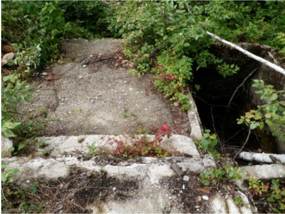
Figure 18: Concrete Tank to Right of the Concrete Slab in Northeast Portion of Stamp Mill Foundation (View East)
