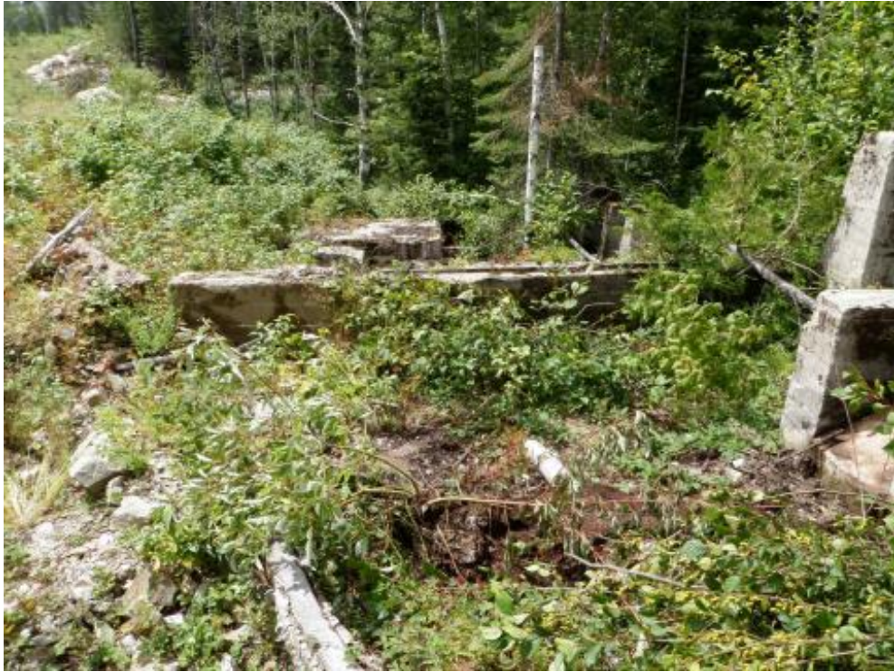
Figure 14: Northwest Corner of the Stamp Mill Foundation Looking along the South Wall of the Structure (View West)
