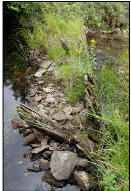
Figure 11: Close Up of Timber Crib Dam Structure, October 2011 (Source Golder Stage 1 Baseline Study and Stage 2 Archaeological Assessment 2013).
