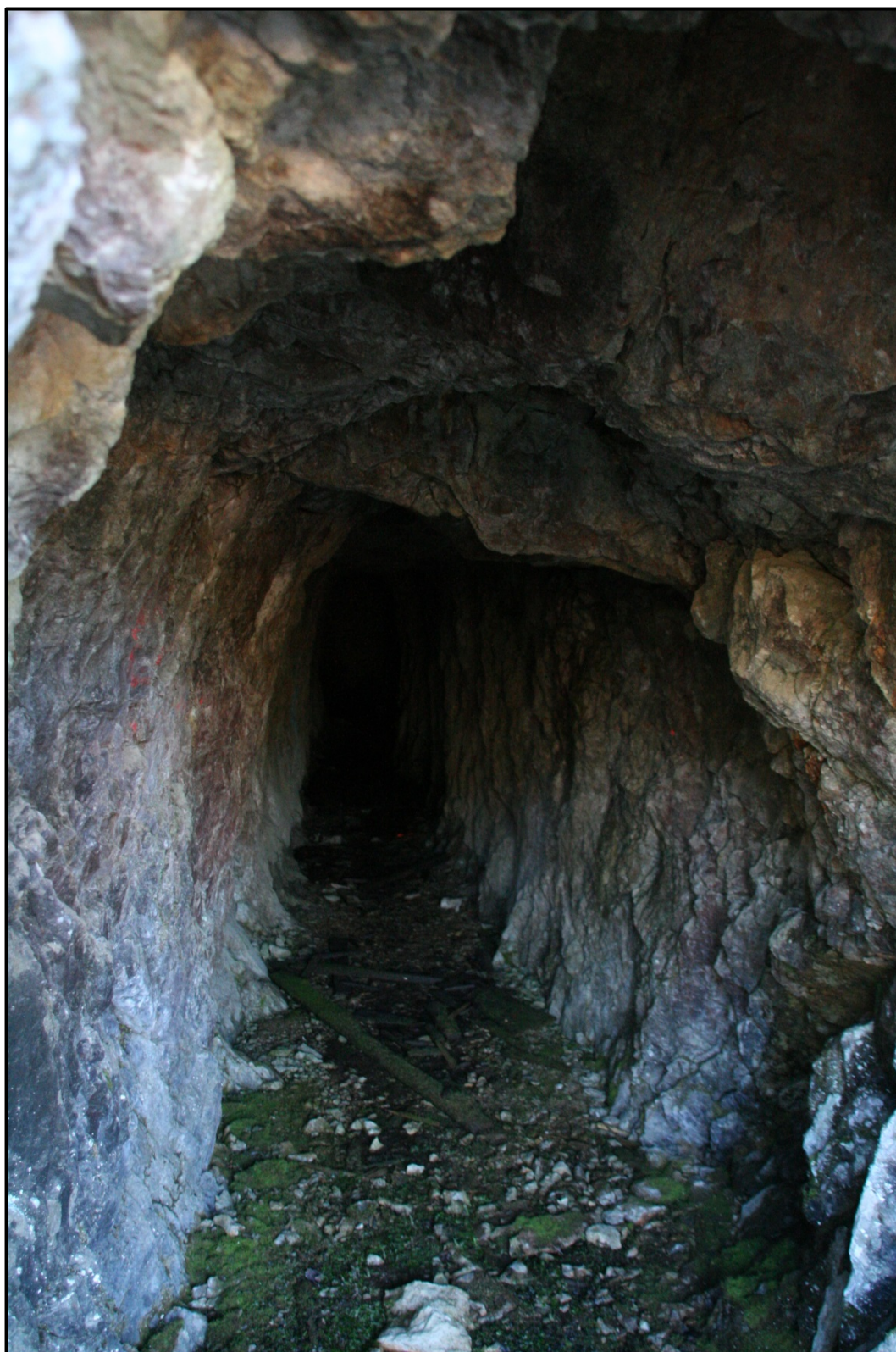
Plate H-4: Adit 2 looking from entrance; the end of tunnel is not visible
