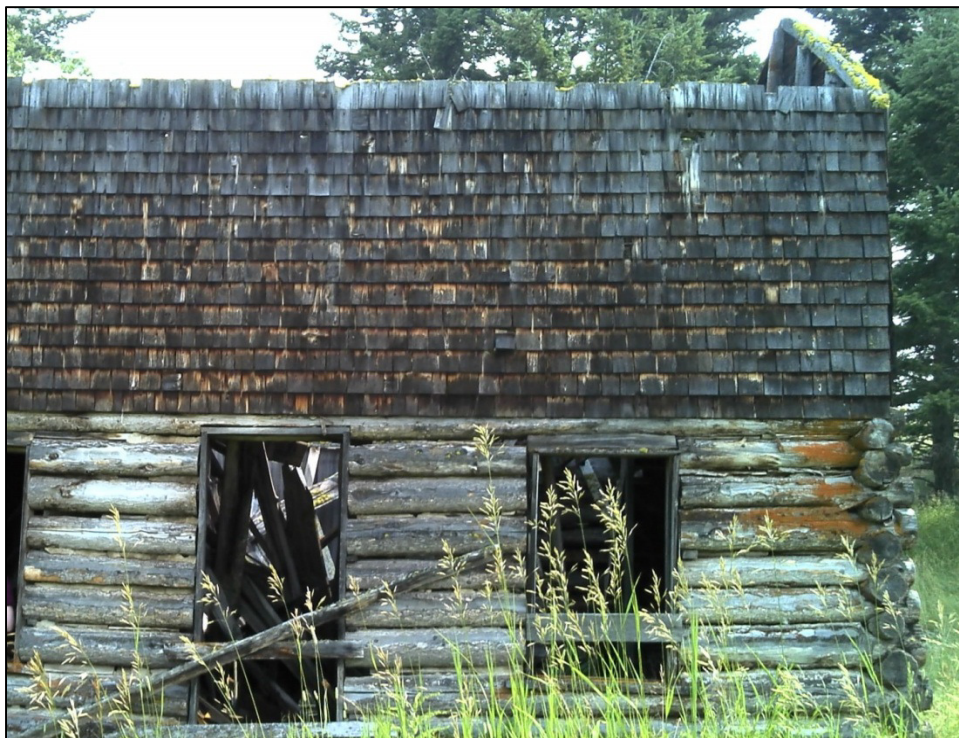
Plate 4.2-1. View of the exterior of the two-storey building on the Gainer homestead, looking south.
