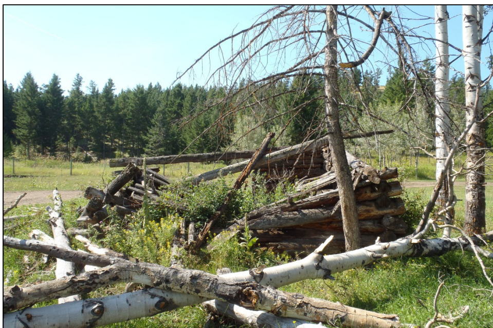
Plate 4.2-11. View south of structure M20-HF1 with collapsed roof.
