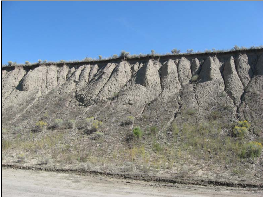
Figure 4.10 Gully Erosion in Cut Slope (WP 98)
